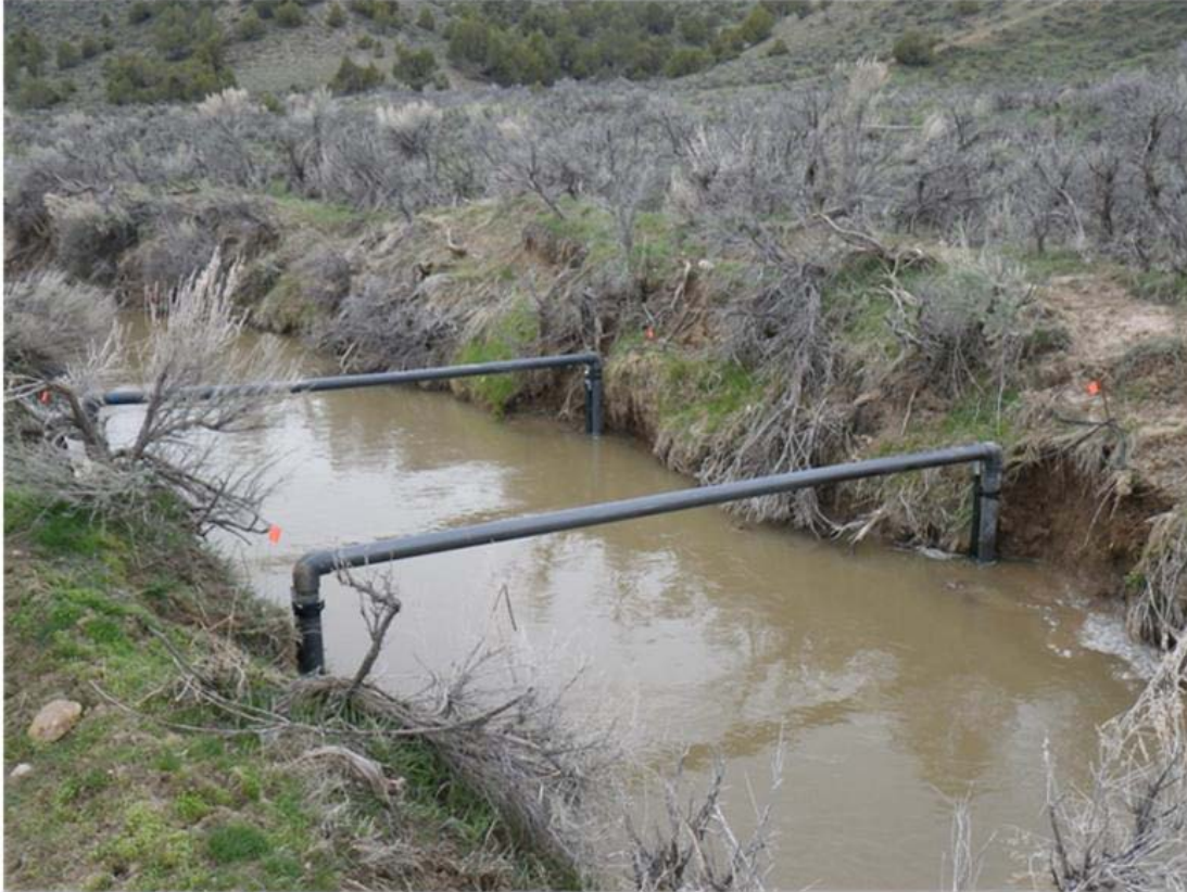
Figure 2. Passive interrogation array in Maybell Ditch near Maybell, CO immediately following installation on April 21, 2011.
